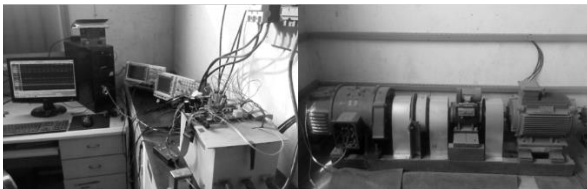
Figure 13. Experimental system of IM driven by three-phase thyristor circuits
