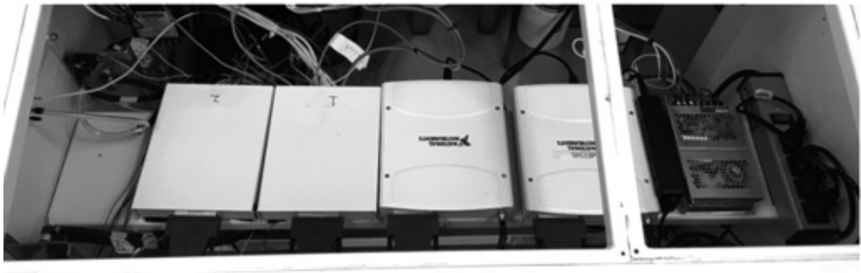
Figure.4 DAQ Components Installed
